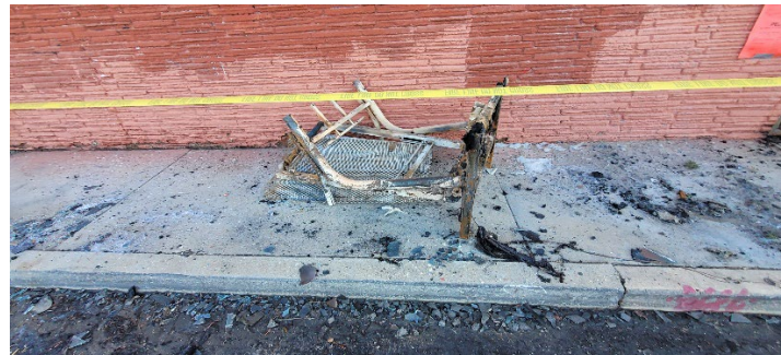
Fallen debris from fire on October 28, 2024, to the sidewalk on North San Fernando Road.
