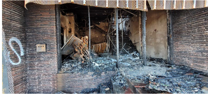
Interior fire damage.
