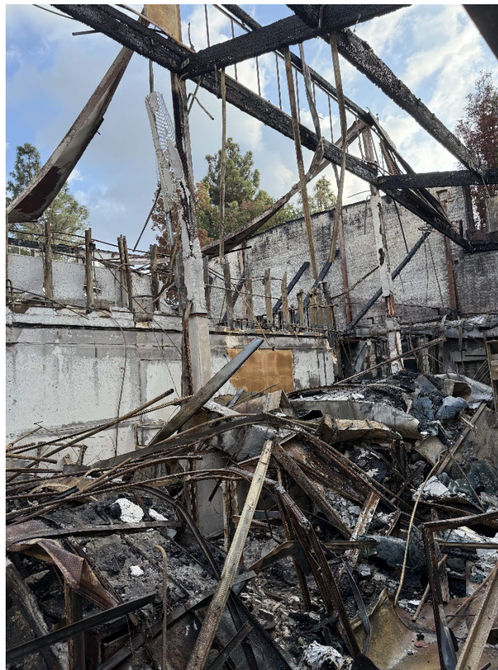
Collapsed steel structure due to the October 28, 2024, fire.
